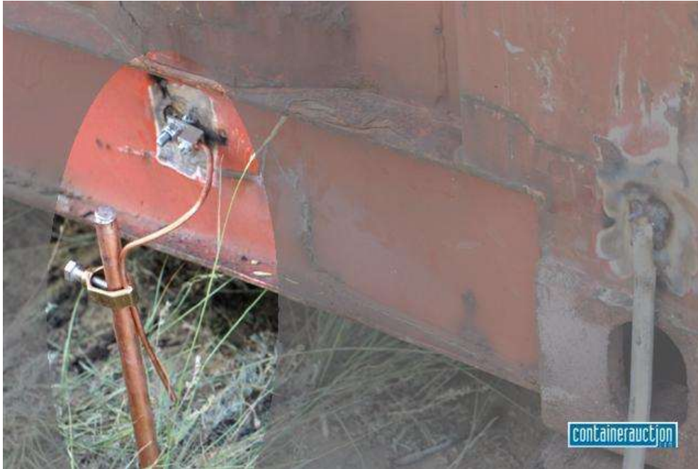
Figure 6: Earthing rod connected to a container
