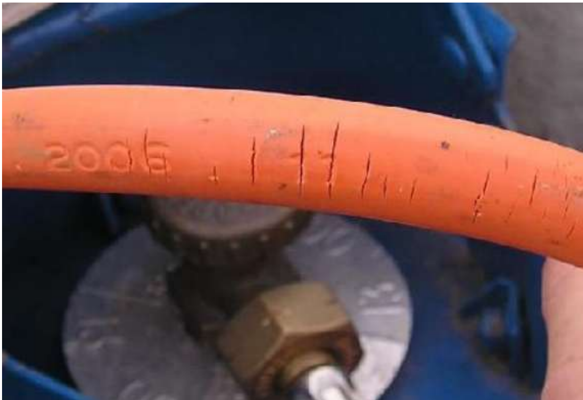
Figure 10: Perished or old hoses will fail inspection
